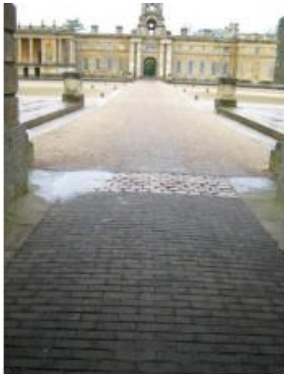
Example of uneven surface
